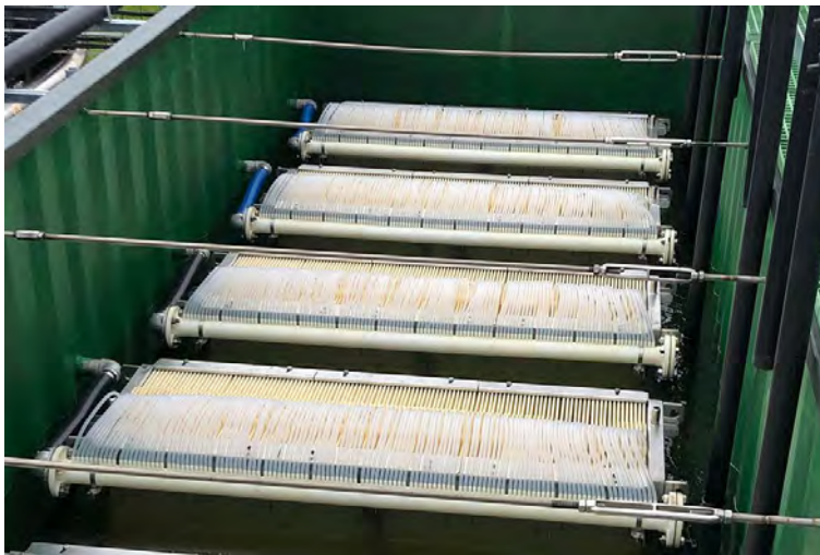
Figure 6: Flat Sheet Membranes Utilised in an MBR
